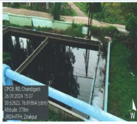
View of Chlorine Tank with outlet of 17.3 MLD STP Zirakpur.
