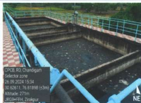
View of floating plastic material in selector zone/anoxic tank of SBR.
