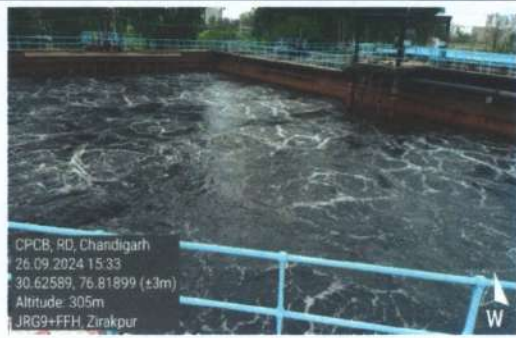
View of SBR Tank 02 of 17.3 MLD STP Zirakpur.
