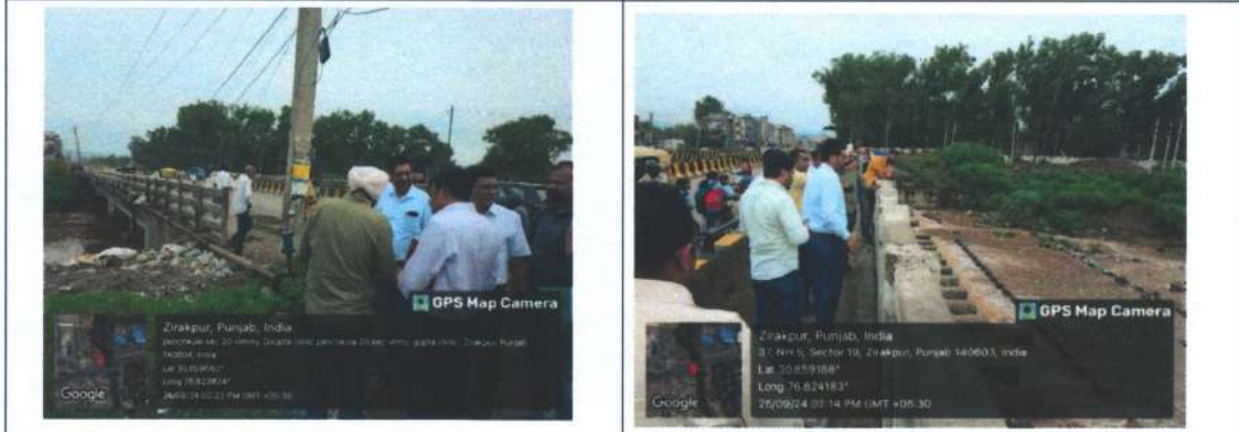
View of Sukhna Choe at Sector 20 Panchkula U/s bridge and Solid waste dumped.
